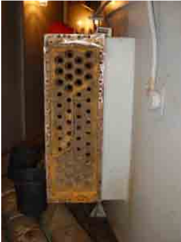
Generator 3 - Air Cooler No. 2
