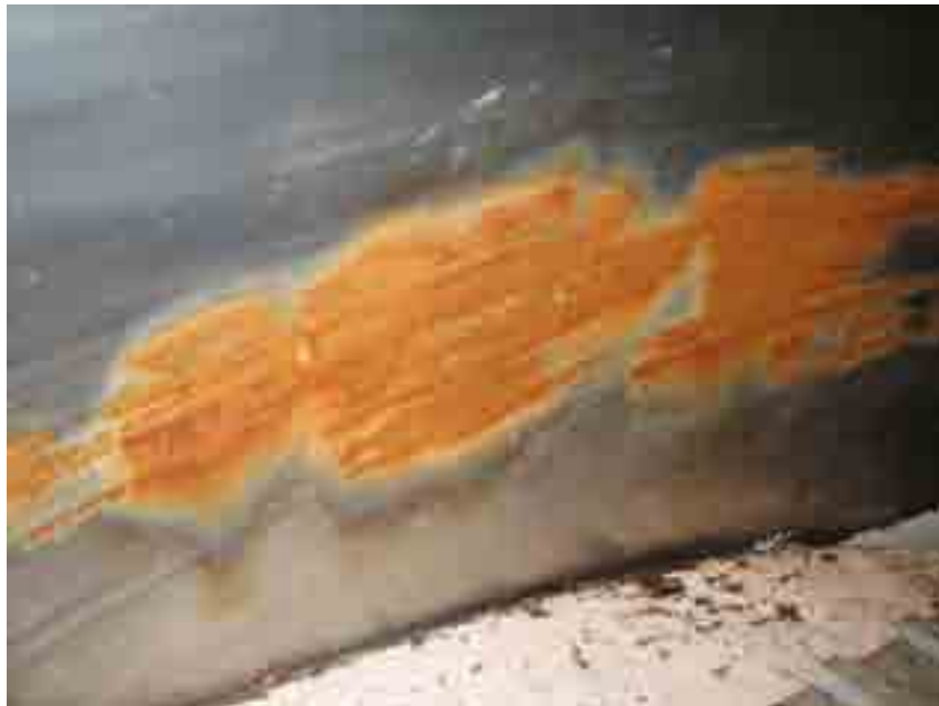
Picture of Turbine Blade Scrape with Liner Notice White-Blue Area on Stainless Steel Liner due to Heat
