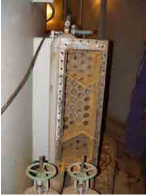
Generator 3 - Air Cooler No. 1
