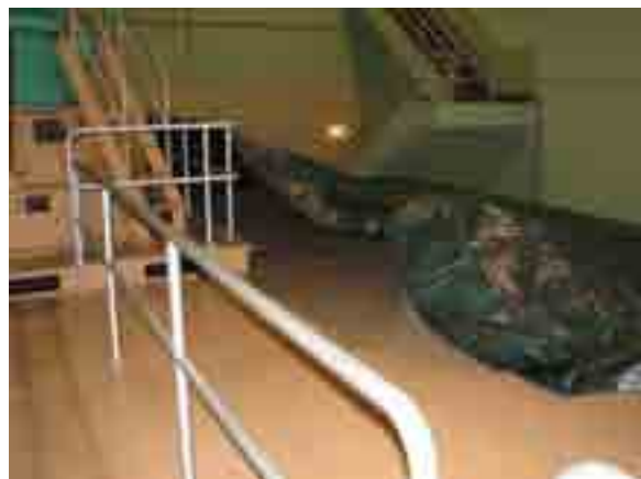
Rain Leaking on Generator Housing
