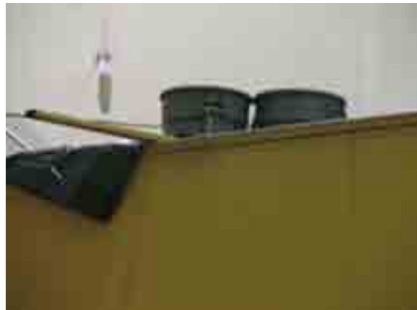
Rain Leaking on Generator Housing
