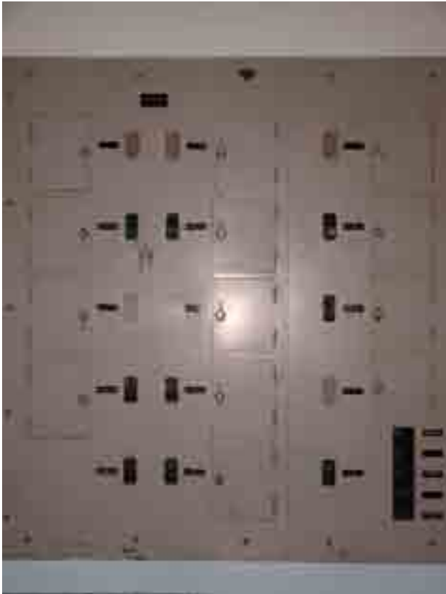
Denison Wall Mounted MCC
