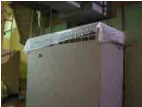
Rain Leaking on Electrical Grounding Cubical
