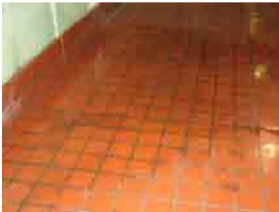
Rain Leakage on Floor
