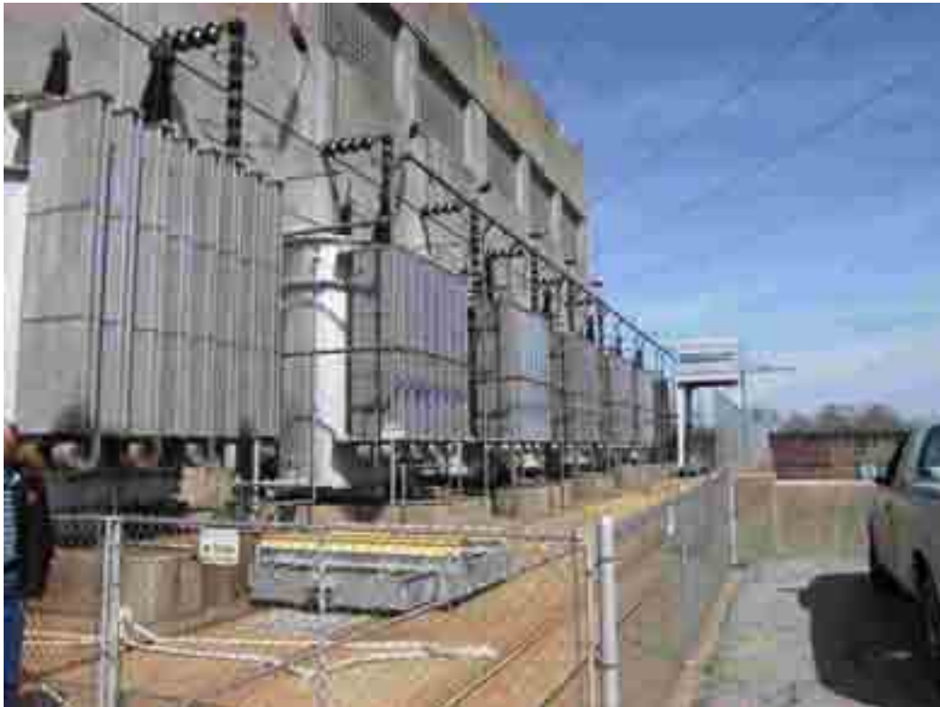
Denison Main Power Transformers
